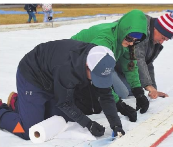
When the liner sheets are where they’re supposed to be, volunteers seal the seams with Tyvek tape.
