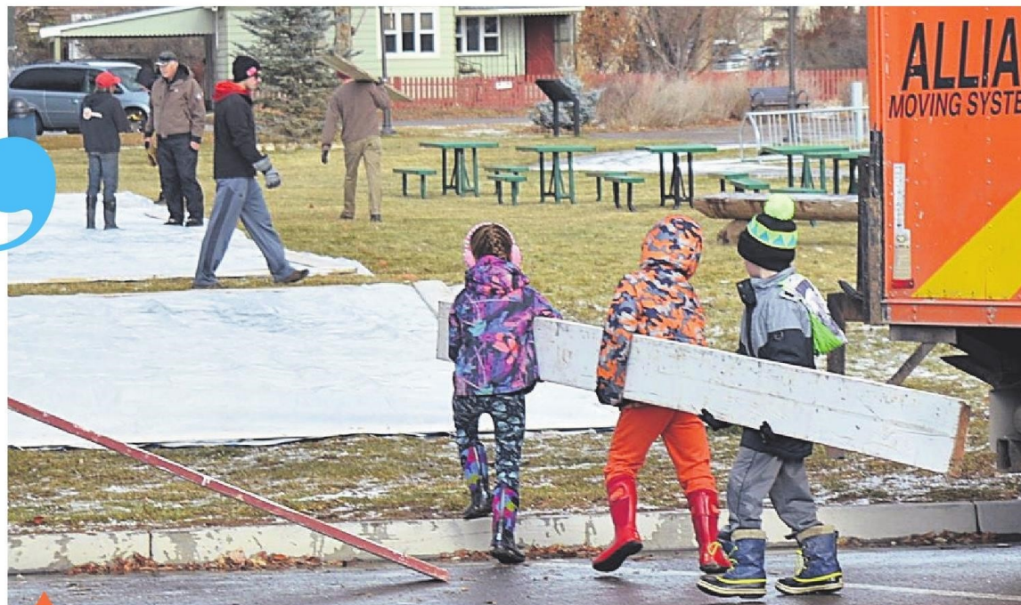
Volunteers of all ages showed up the Friday after Thanksgiving, as they always do, to help build the Tom Ehrenberg Memorial Ice Rink in Eagles town park. Volunteers started building the rink every year beginning in the 1930s, when Eagle built its town park.
